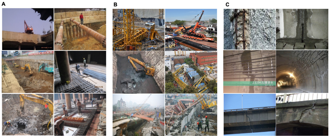
Fig. 1. Examples of (A) unsafe behavior; (B) unsafe plant; (C) structural defects.
